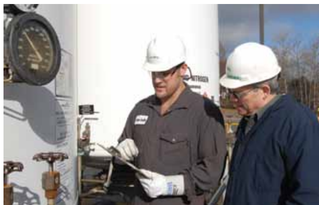
▲ Figure 1. Gaseous nitrogen, vaporized from onsite liquid storage into a local distribution system, is used for a wide variety of applications, including blanketing, inerting, purging, stripping, and sparging. Other supply modes ranging from cylinders to onsite generation are also used to deliver nitrogen gas.
