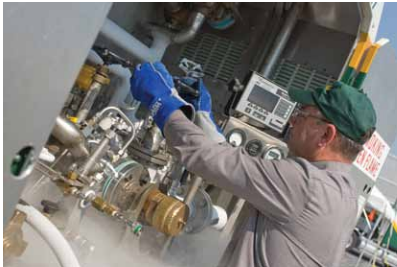
► Figure 3. Cryogenic tankers and liquid cylinders are equipped with pressure relief valves to allow the product to periodically vent due to pressure buildup. While this venting is normal and safe, it should always be done in a well-ventilated area to avoid creating an oxygen-deficient atmosphere.
